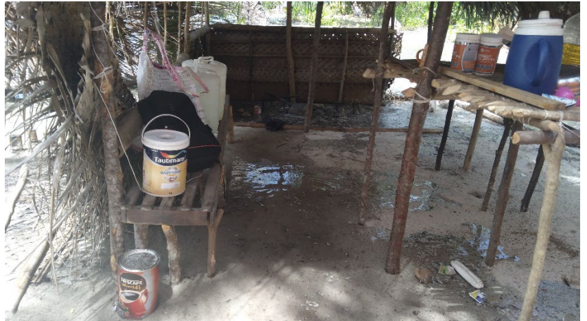
Figure 53: Flooding at camp kitchen after storm surge and severe weather
